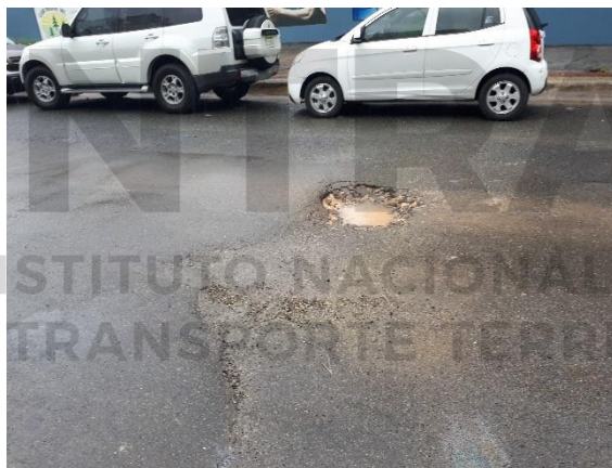
Av. Winston Churchill /Calle Francisco Carias Lavander
